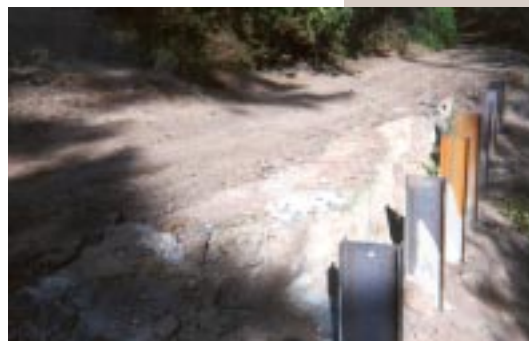
Figure 4 The affected road was regraded. Temporary piles were left in place.
