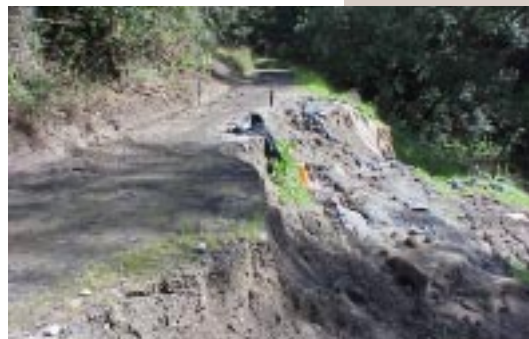
Figure 1 The landslide on Meters Road threatened a concrete water pipe buried under the road.
